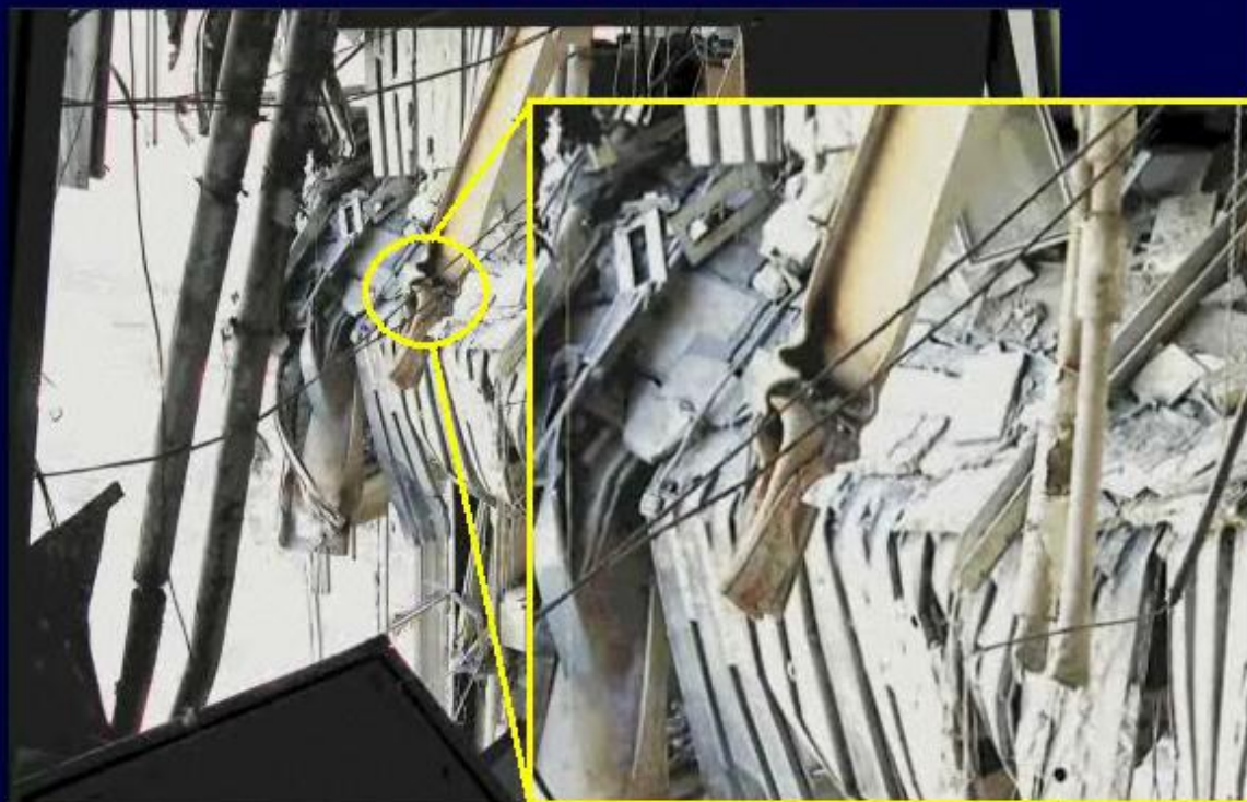
Figure 6-10 Area of collapsed floor slab in bays between C-8, E-8, C-7, and E-7, from the 15th floor.
